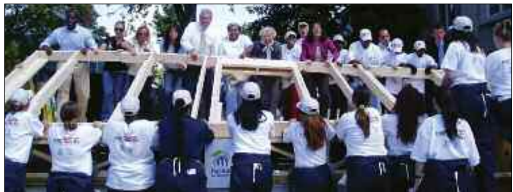
Gov. and Mrs. Carcieri help raise the first wall at the Women Build/Lowe's house on Potter's Avenue.
