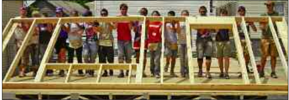
May 12, 2007: The first wall goes up for the third Bike & Build house, located at 17 Handy St.
