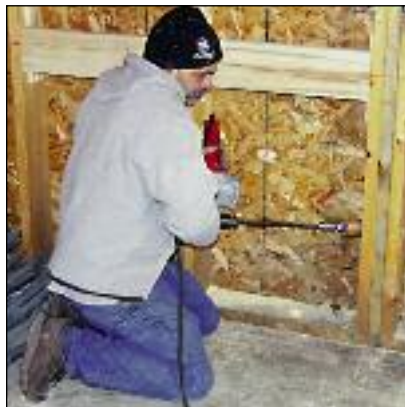
Winter work: Plumbing (left) and electrical work (right) begin in Feb., out of the cold and wet weather. The work went on as shown here on Veazie St., as well as at the Jefferson St. site in Pawtucket.
