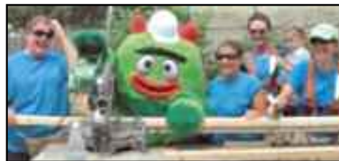
Brobee of Yo Gabba Gabba works on site with a miter saw with volunteers from Dermatology Professional Inc. on Trask St.
